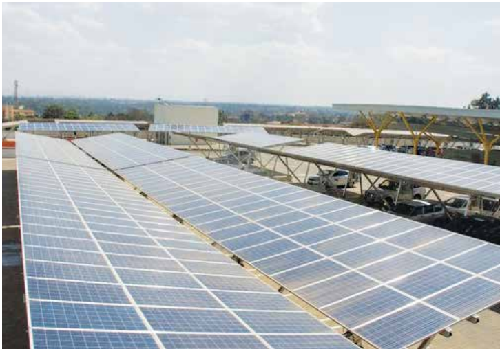
The carport at the Garden City mall is fitted with multiple solar panels that help cut electricity costs. Below; UNEP's headquarters in Nairobi.
